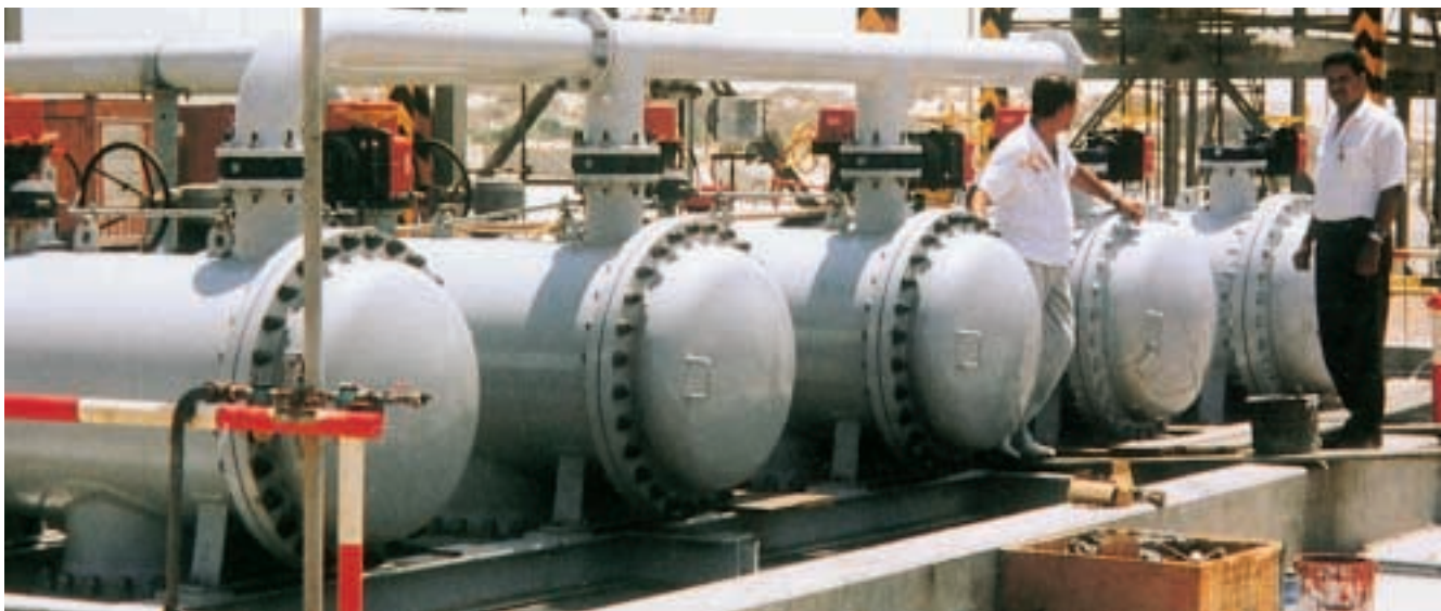
Fig 2. Five Alfa Laval Filters in parallel serve as main inlet cooling water filters for an ammonia plant on the Mediterranean Sea.
